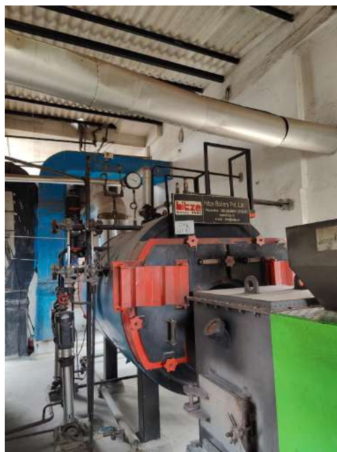
CNS biomass boiler at Remedix Pharma Pvt. Ltd.
